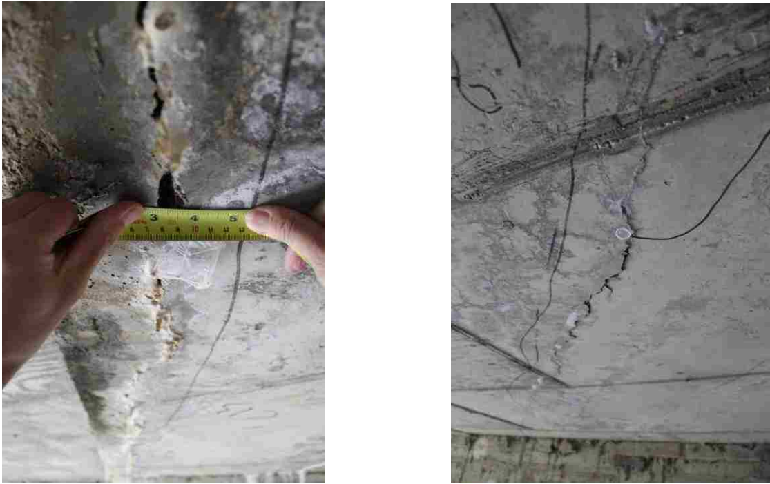
Figure 5.14. The cracks of span 1
