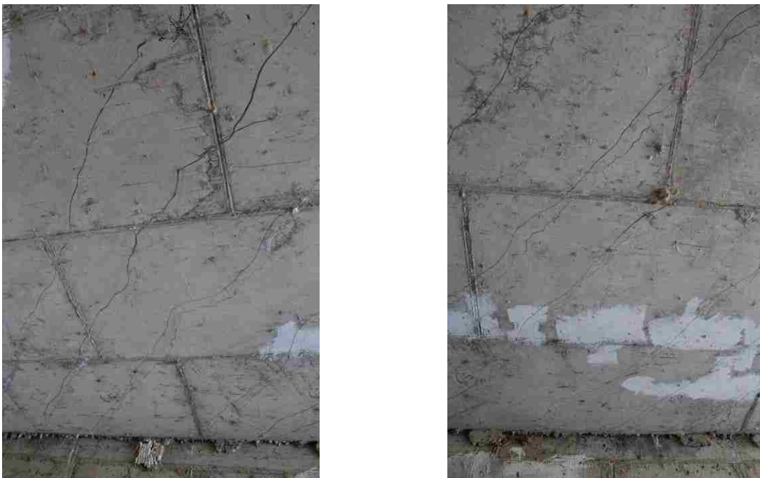
Figure 5.17. The cracks of span 4
