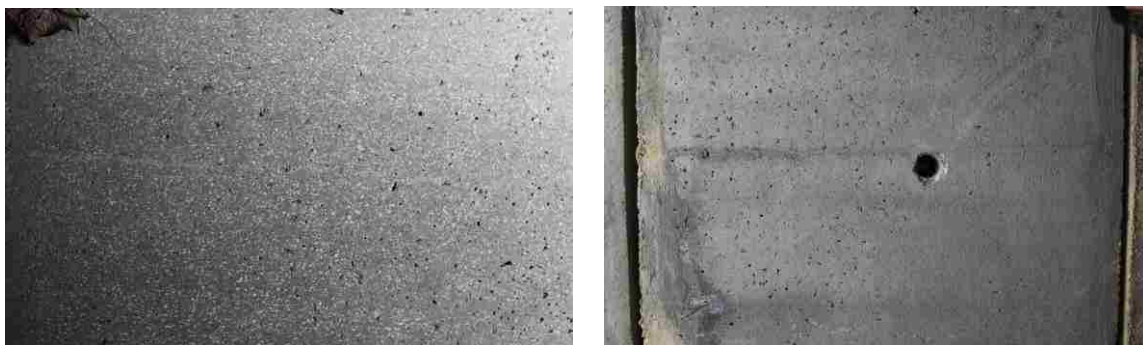
Figure 5.27. The cracks on the top (left) and bottom (right) of Box 2
