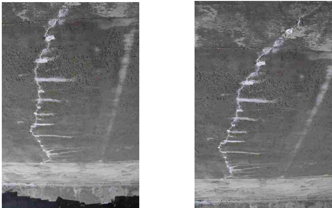
Figure 5.19. The cracks of span 6
