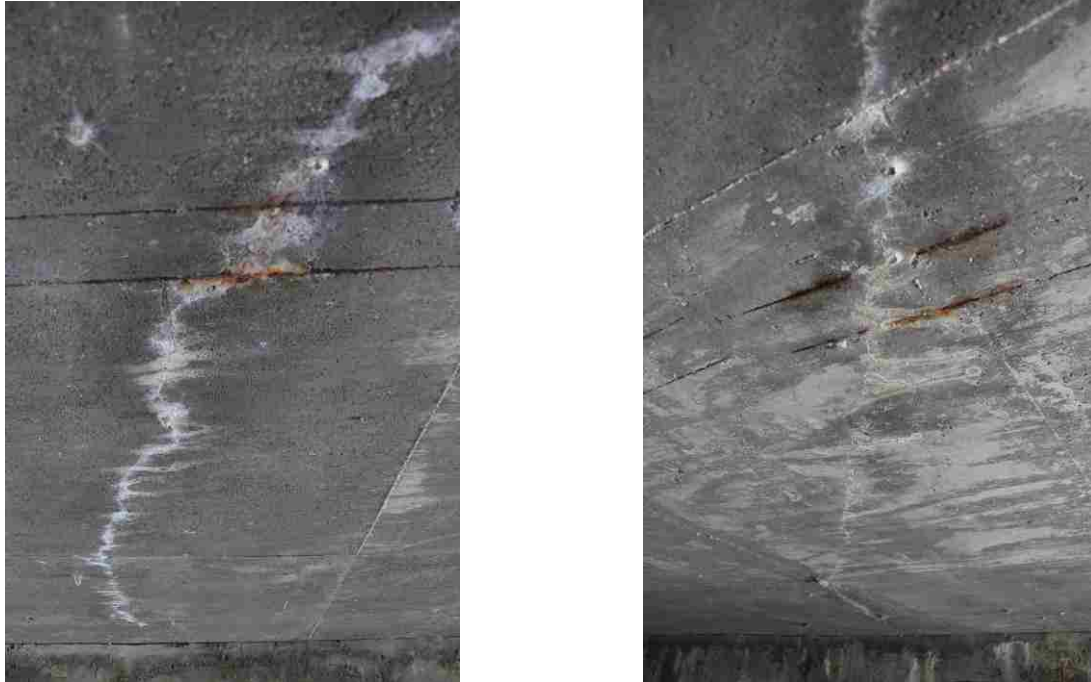
Figure 5.18. The cracks of span 5
